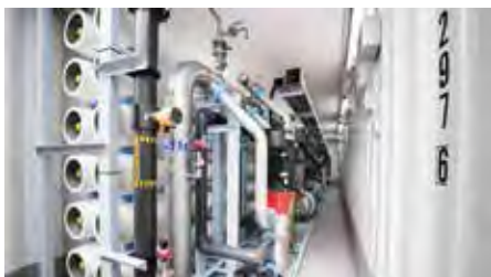
SWRO System Container
