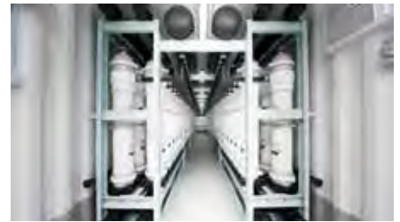
Pre-treatment UF System Module Container
