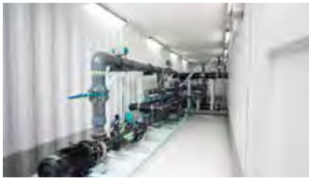
UF Valve Rack Container
