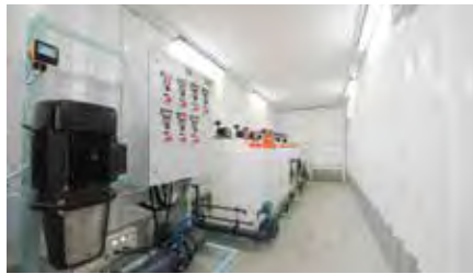
Chemical & CIP System Container
