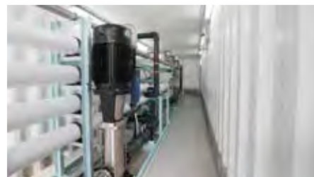
BWRO System Container
