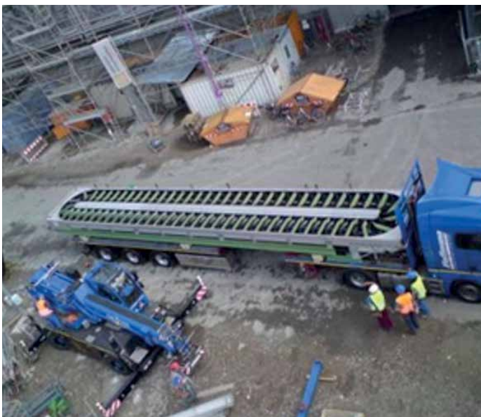
GKM 9 Power Plant, Mannheim, Germany
