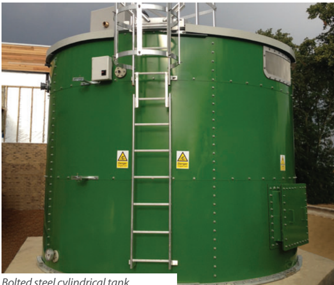
Bolted steel cylindrical tank
