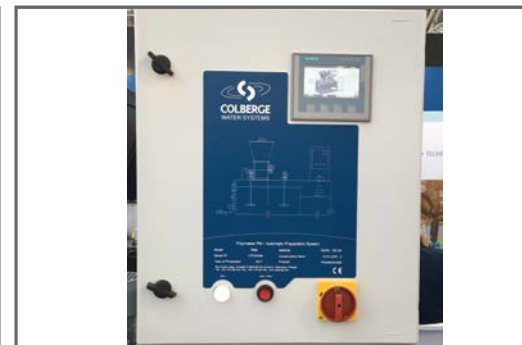
Control panel featuring Siemens PLC & HMI
