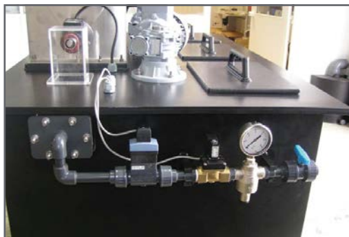
Dilution water inlet line
