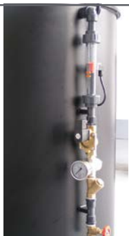
Dilution water inlet line
