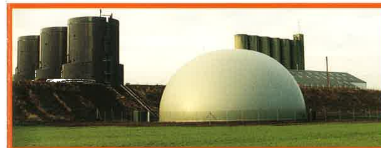
Double membrane gasholder
