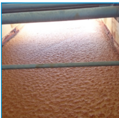
DAF retrofitted with MicroGas™
